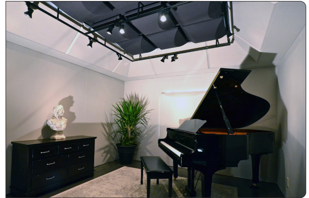
Custom fabric Hemispheres installed at Yellow Hammer Studio - Photo courtesy of Carl Tatz Design
