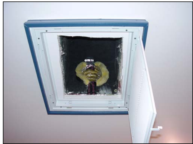
Figure 4.6b — Silent duct boot, grille open
